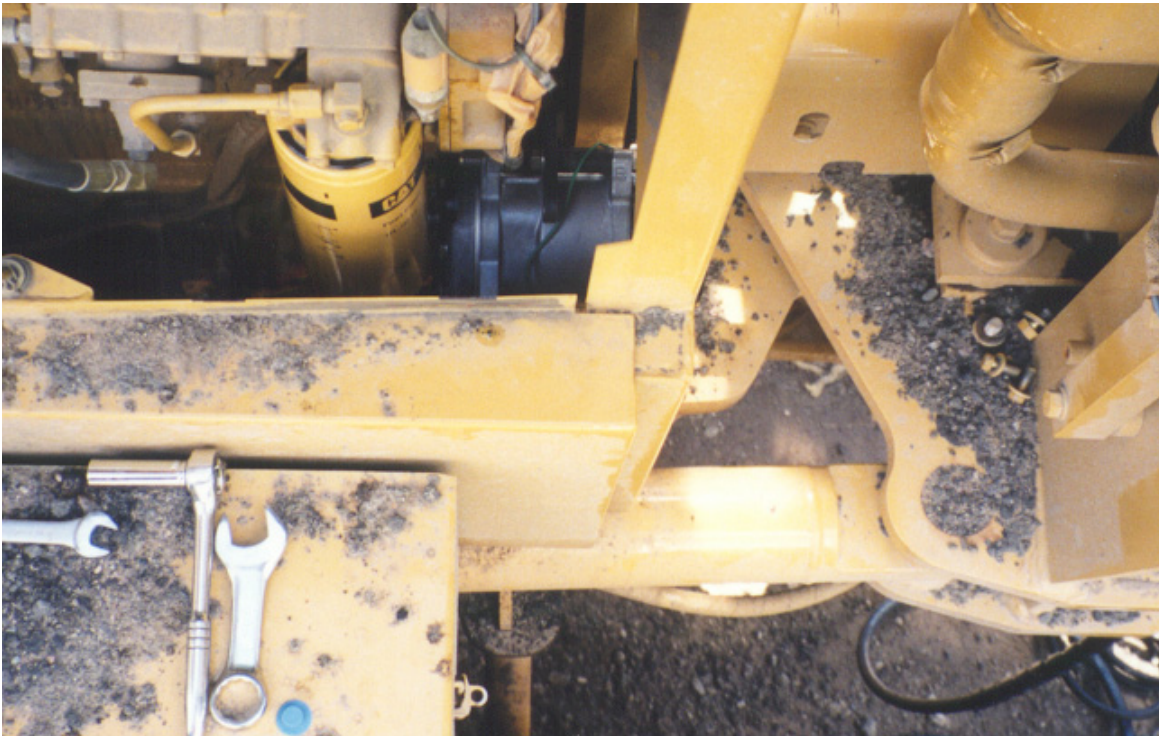
Compressor mounted in location on engine.
