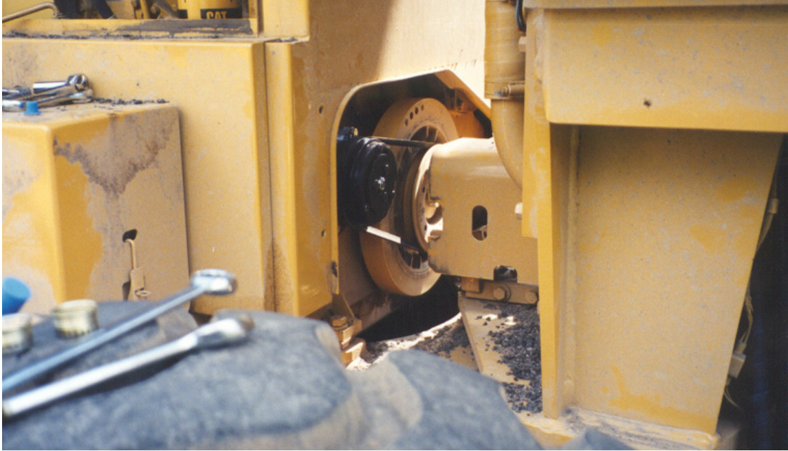
Compressor showing drive assembly.
